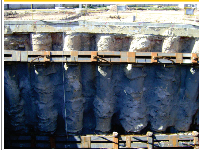
Figure 1– Example of application of circular cross section elements of reinforced concrete working as beams in a retaining structure (Maffei, (8))
