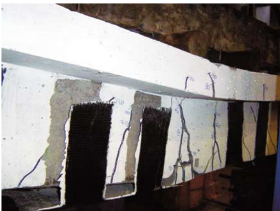
Debonding of CFRP – VTF2
