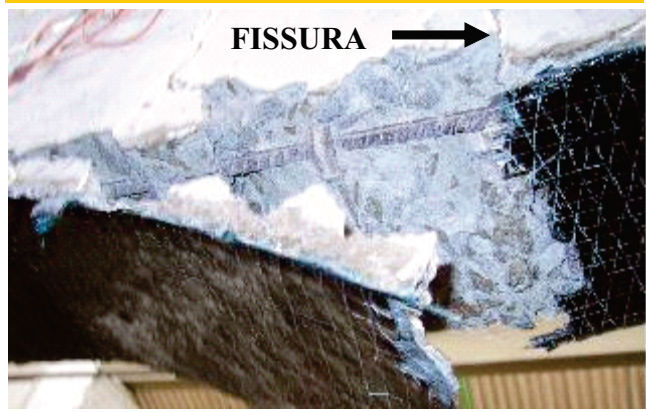
Figure 5 – Rupture of FRP close to a flexural crack tip
